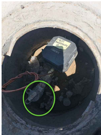
Type of Supply Piping Material: PEX
